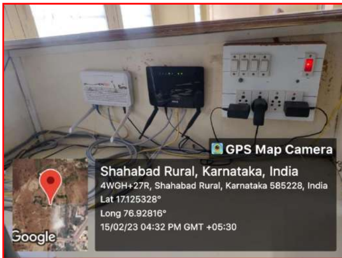
Fiber Optics Internet connection in Office
